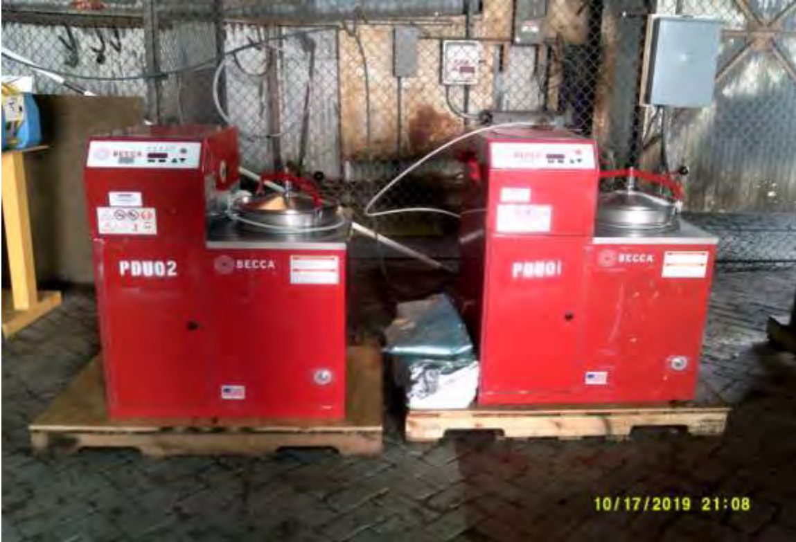
P-1 NEW SOLVENT DISTILLATION UNITS INSTALLED IN PAINT SHOP
