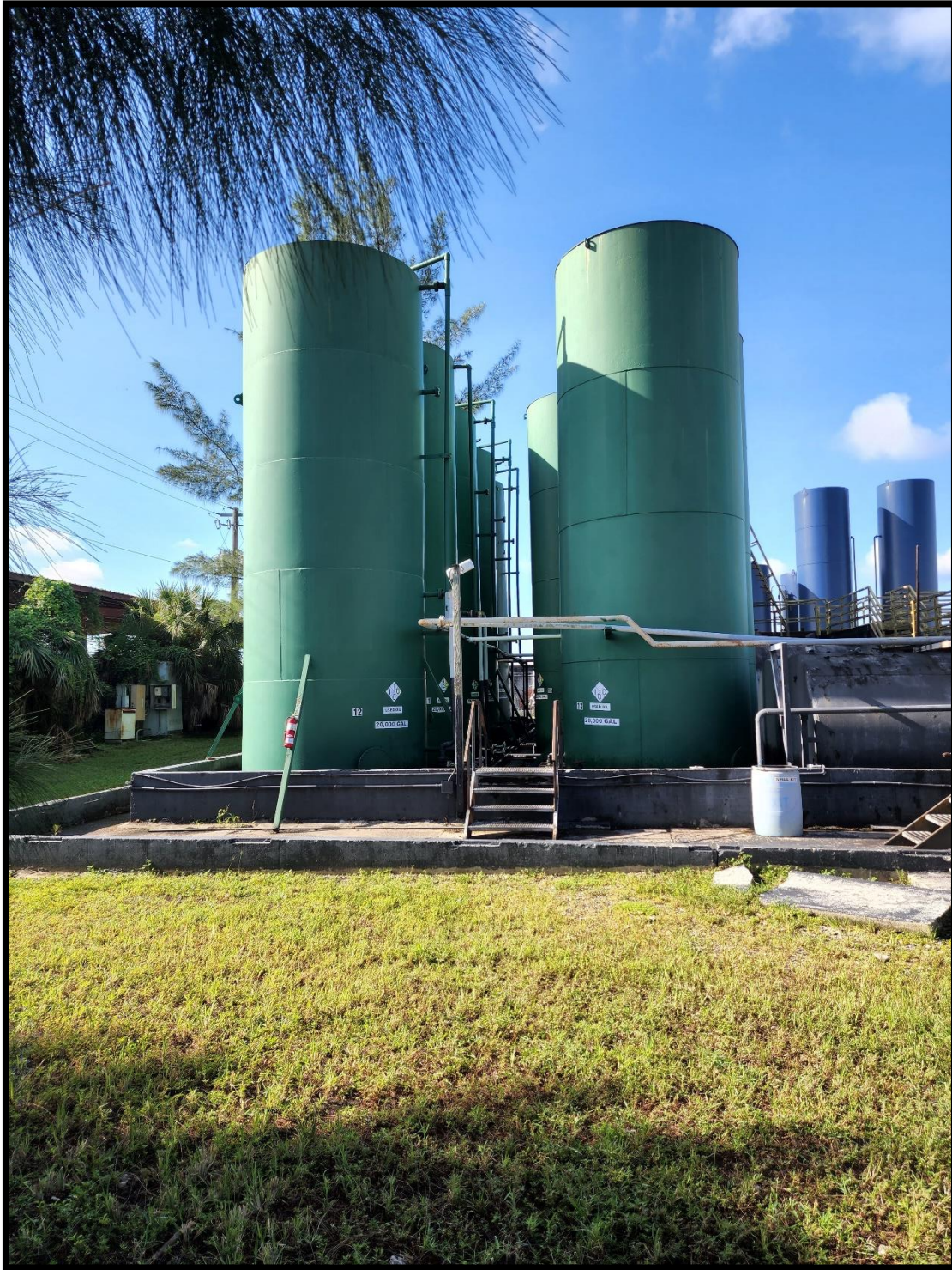
Photo 7: Vertical Aboveground Storage Tanks with Secondary Containment #1 (View from the North)
