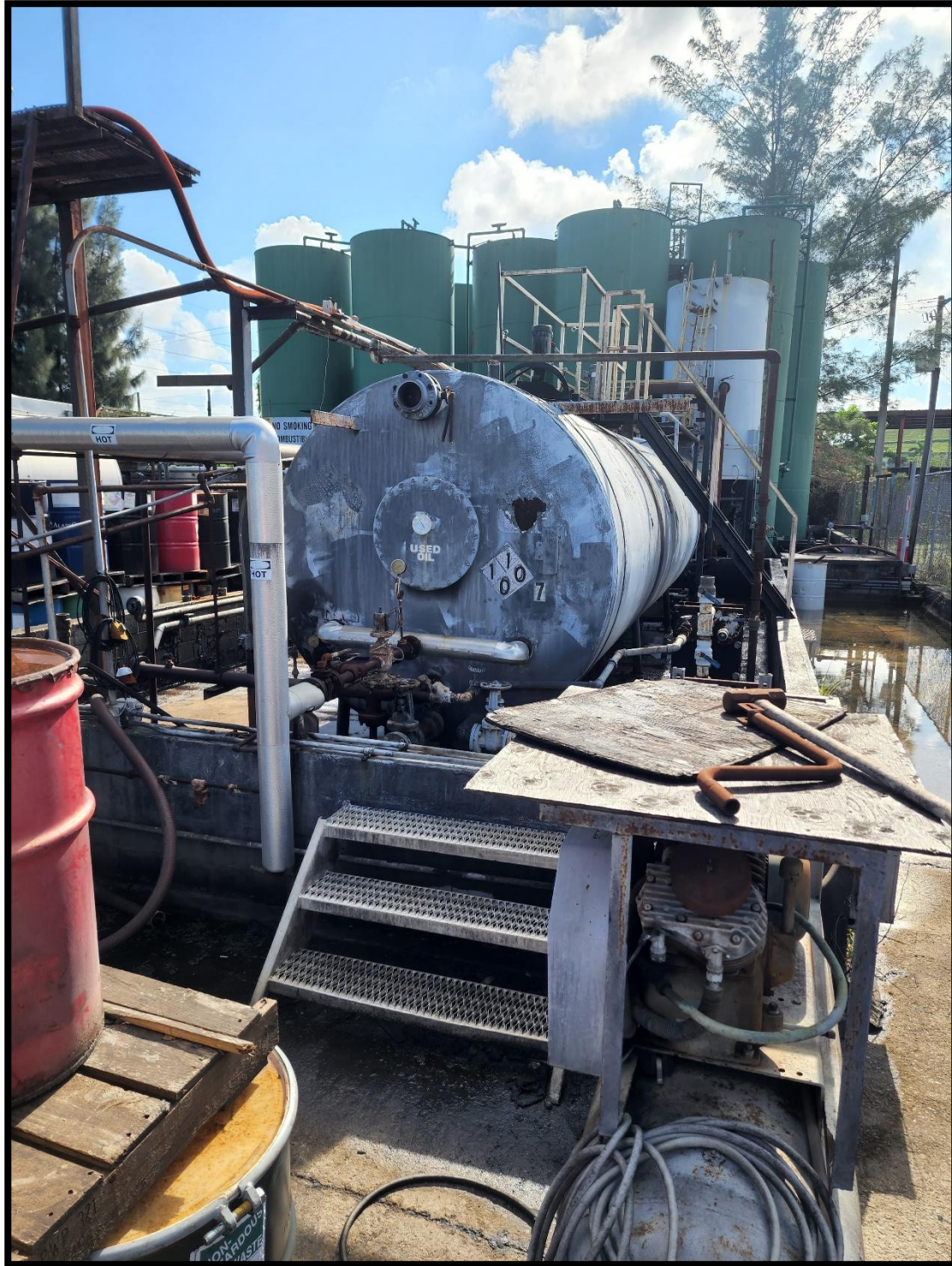
Photo 12: Tank 7 in Secondary Containment #2 (View from the West)
