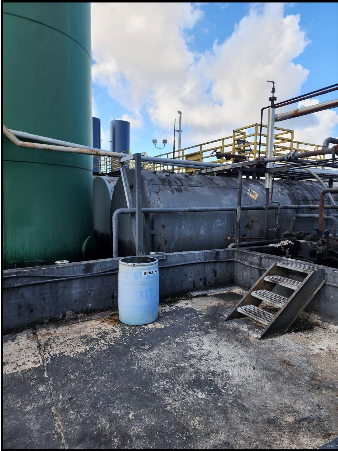
Photo 9: Horizontal Aboveground Storage Tanks in Secondary Containment #1 (View from the North)
