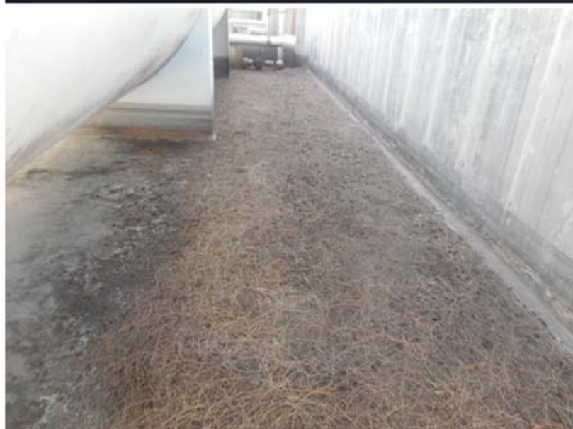
CONTAINMENT AREA NEAR HORIZONTAL TANK EXCESSIVE DEPRIS
