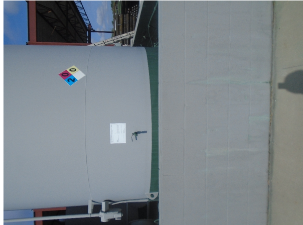
Photo 28-Hazardous waste release from tank farm 2nd containment
