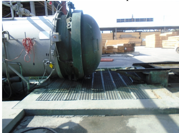
Photo 2 - Cylinder door and sump
