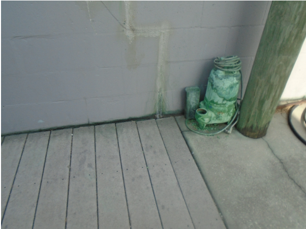
Photo 27-Hazardous waste release from tank farm 2nd containment
