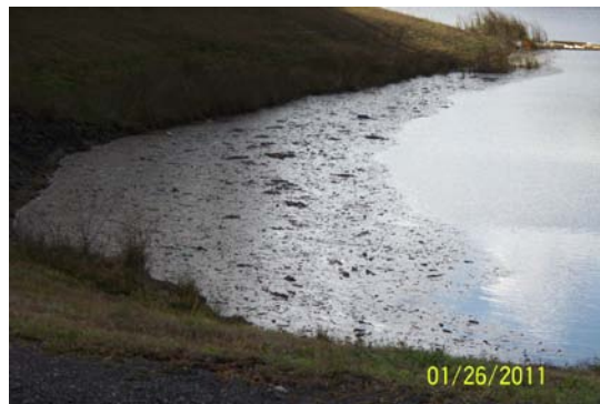
(Northern Section of SW Pond 2 With Minor Debris)
