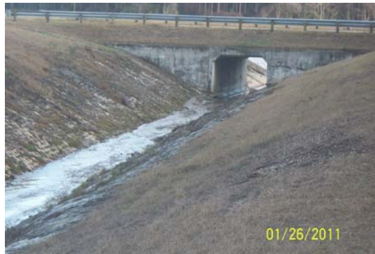
(Stormwater Conveyance System Located on Southern Section of SW Pond 2)
