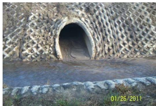
(Sediment in Stormwater Pipe Along Southern Slope)
