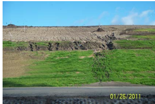
(Erosions Along Southern Slope of Landfill)
