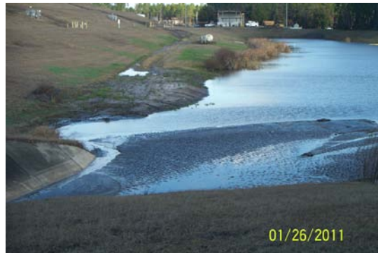
(Southern Section of SW Pond 2 With Deposited Sediment)
