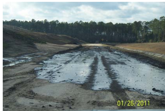
(Erosions Along Western Slope of Landfill)
