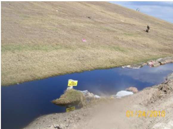
Leachate in Liner "Jog" Area
