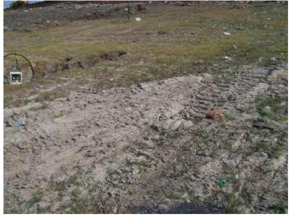
Leachate Seepage Repair Area
