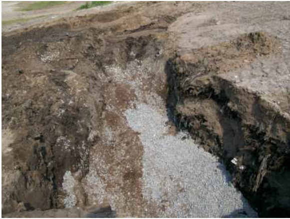
Excavated Seepage Area
