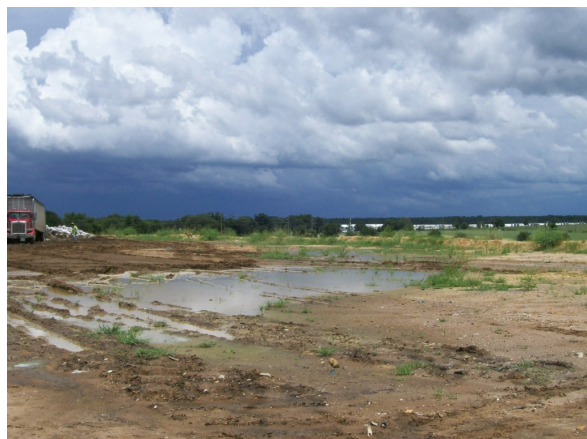
Ponding in traffic area
