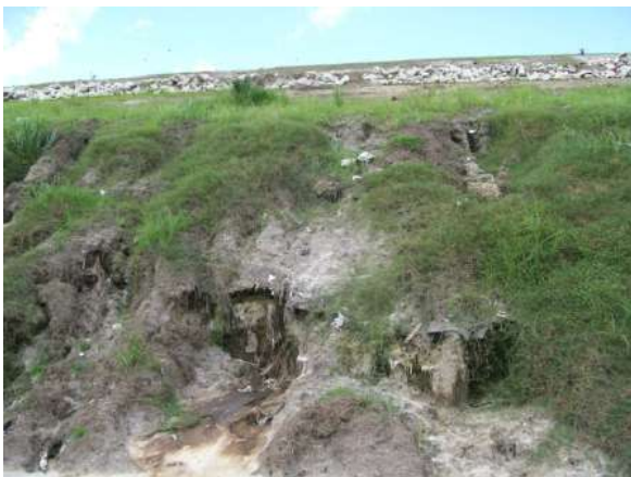
Eroded Slopes Above Toe Drain
