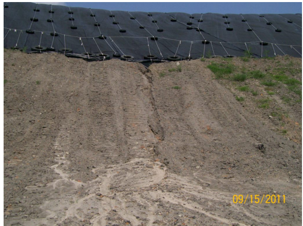
protective soil erosion
