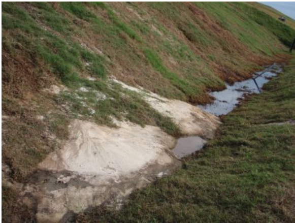
Toe Drain Sedimentation Area
