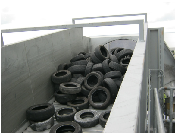
Tire conveyor from truck hopper
