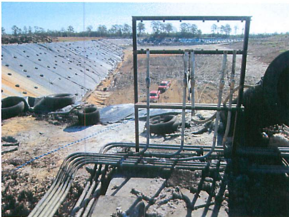
Photo 8: Date: 3/14/2013 Phase 3 detection pump riser controls.
