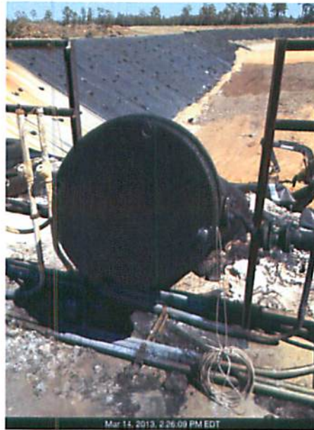
Photo 7: Date: 3/14/2013 Phase 3 side slope riser 24" diameter pipe.
