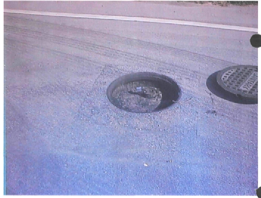
4) Paved CDA – MW-2 located in a manhole on the paved pad.
