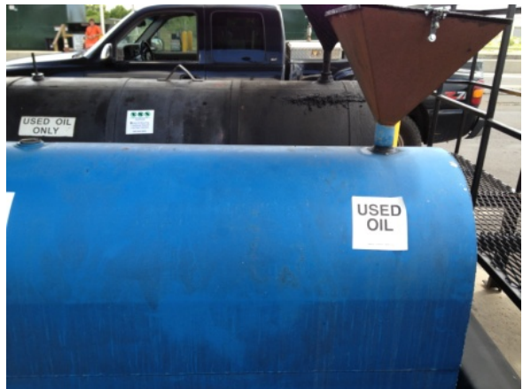
Used Oil Storage
