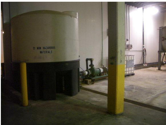
chemical tank in process area
