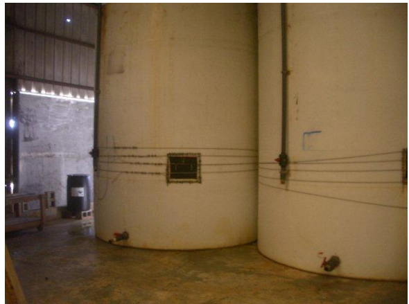
product storage tanks
