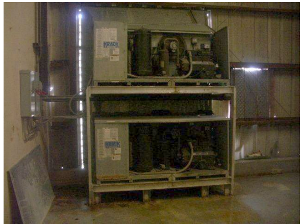
air handler in tank room
