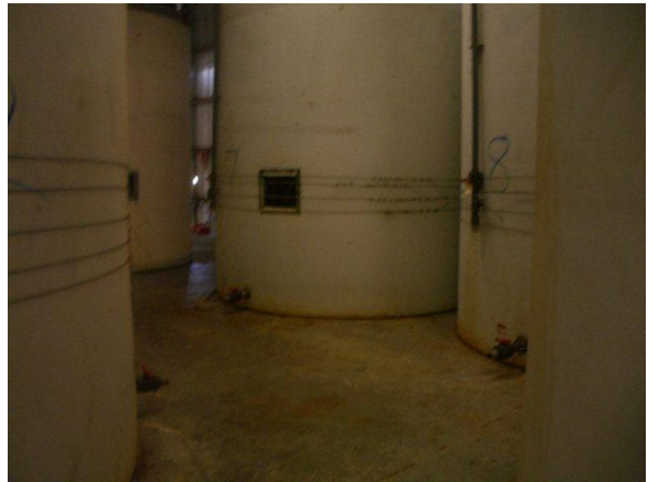
product storage tanks
