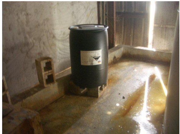
sulfuric acid drum in tank room
