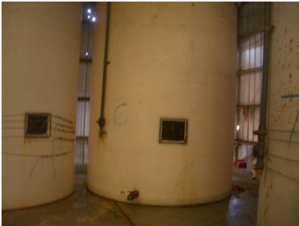
product storage tanks
