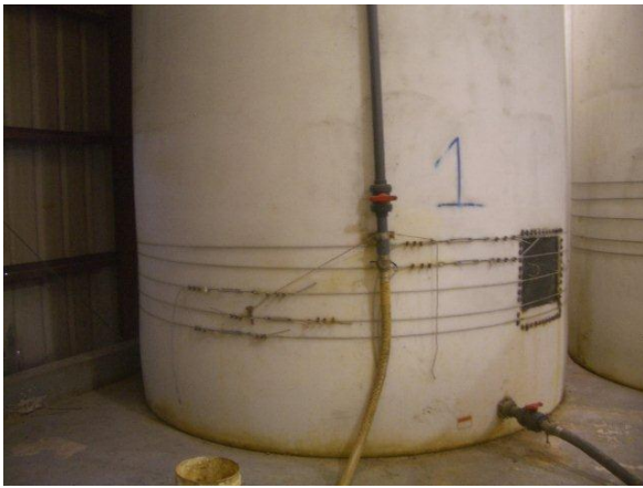
final product holding tank room
