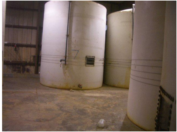
final product holding tank room
