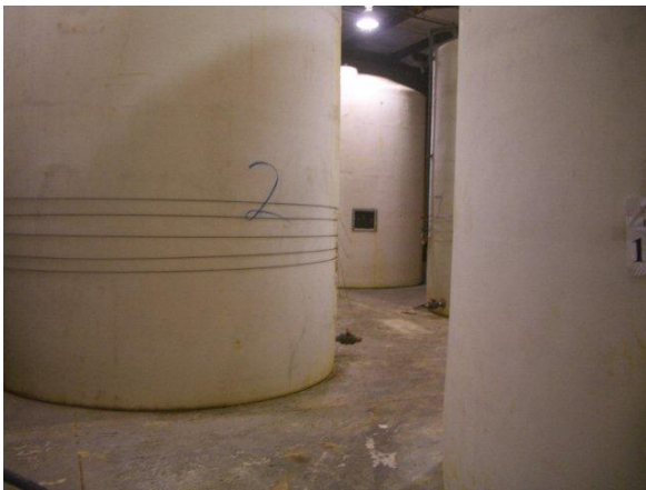
final product holding tank room
