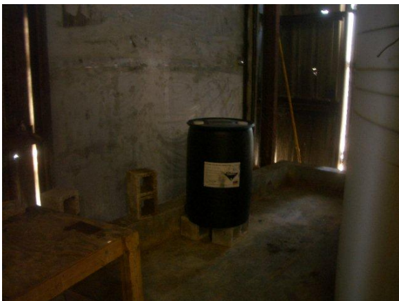
full drum labeled sulfuric acid
