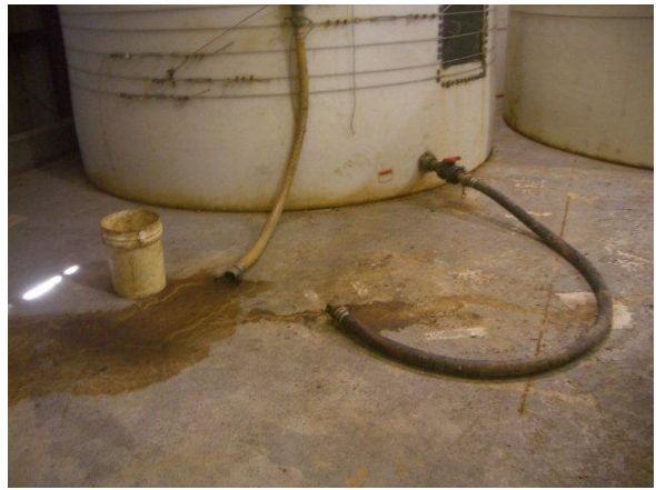
final product holding tank room
