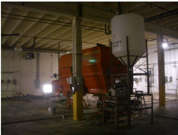
remaining process equipment
