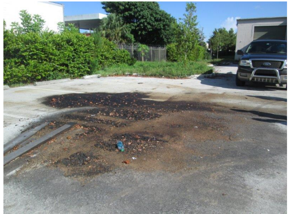
granular residue in parking
