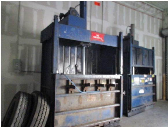
two waste tire balers, west wall
