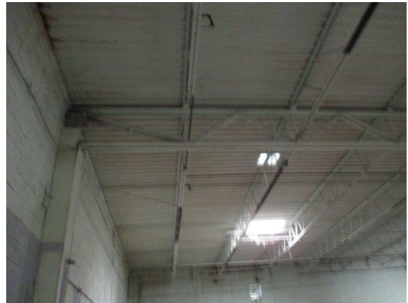
ceiling with fire sprinklers
