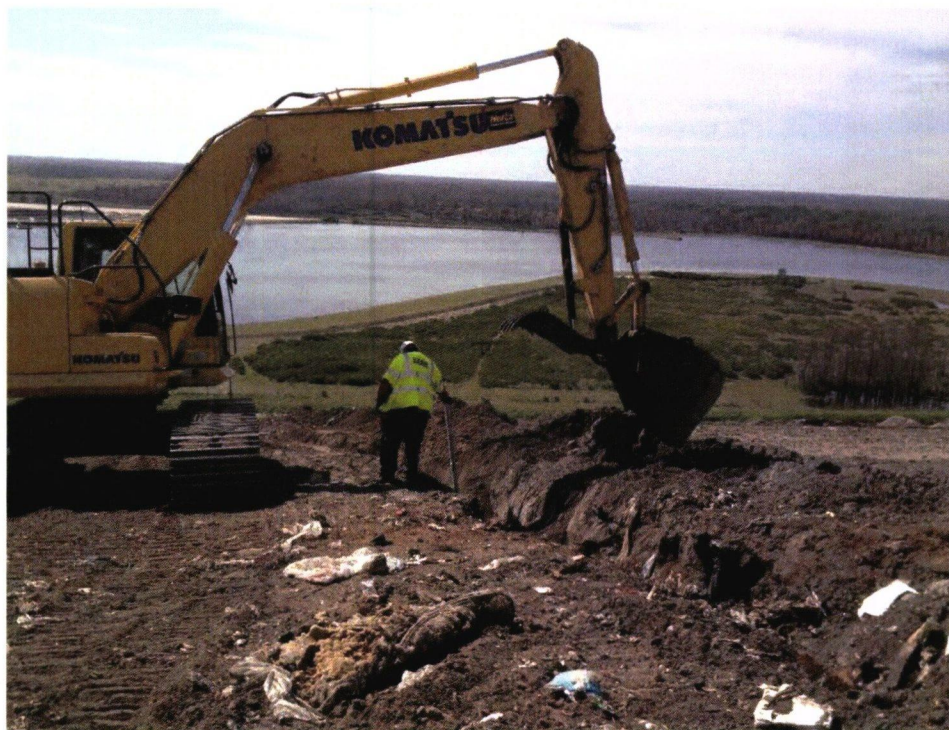
Photograph 23: Backfilled trench. Caution tape applied and survey posts every 50' and at points of interest (typical).
