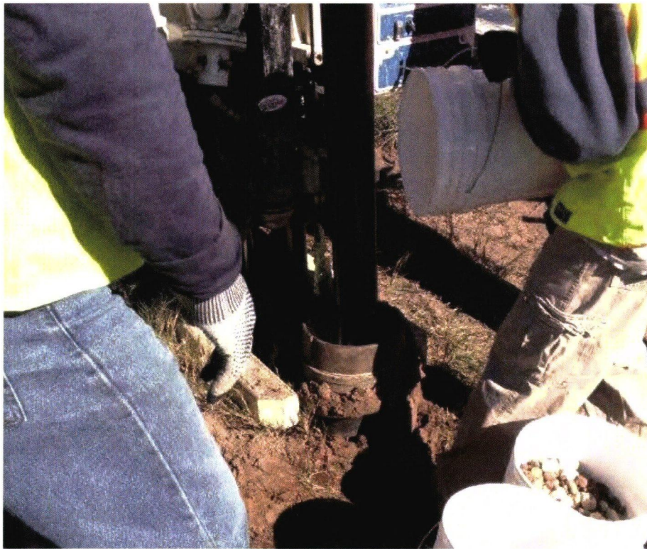
Photograph 47: Installing rock from bottom of borehole to 1-foot above top of slotted pipe (typical).
