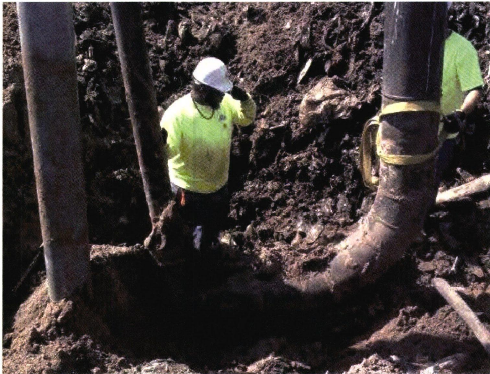
Photograph 28: Existing 90° bend and 12" subheader riser at GW-70.
