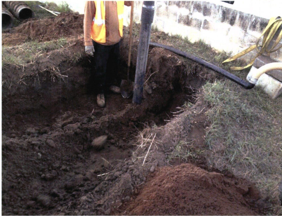
Photograph 48: Excavation of final cover soil to top of liner after well installation (typical).
