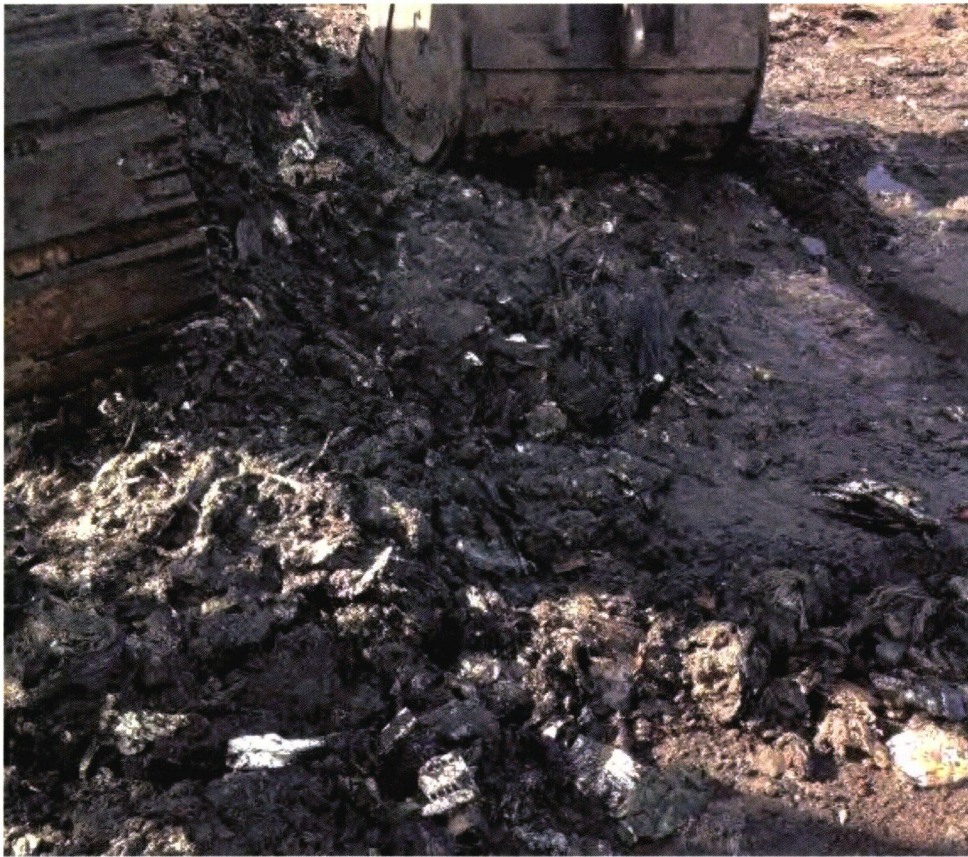
Photograph 7: Saturated waste at bottom of boreholes for top tier wells.
