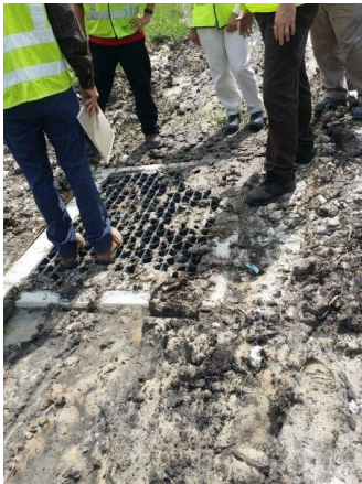
Plugged up grate
