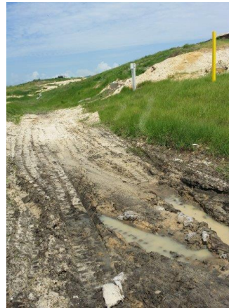
Cell 3 side slope washout
