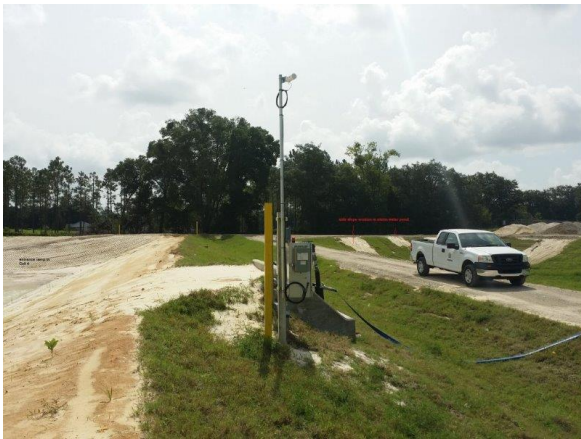
Stormwater pond sideslope erosion
