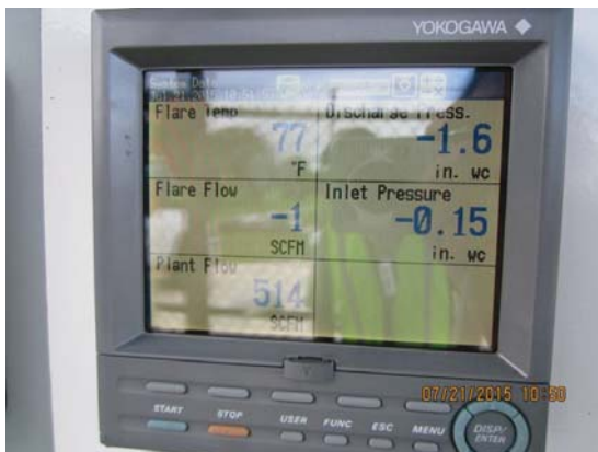
GCCS offline for minor repair
