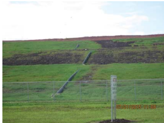
Stage III Erosion to be Repaired
