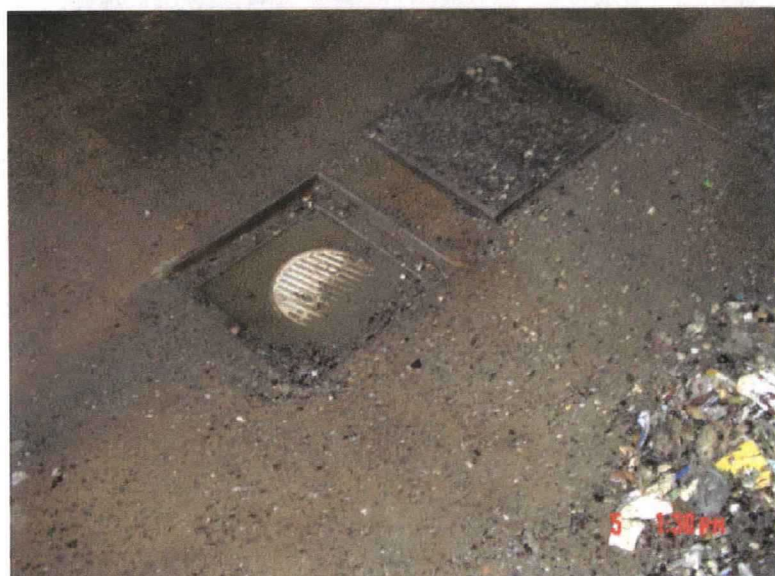
32. Leachate drain inside of MRF
