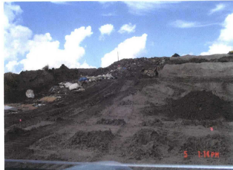
19. Loose waste working face/no berm
