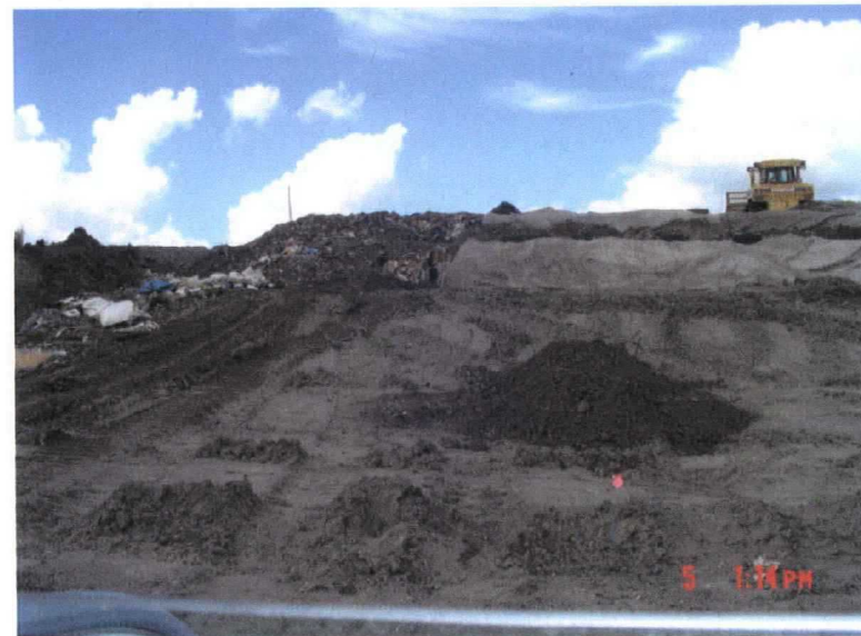
20. Loose waste working face/no berm
