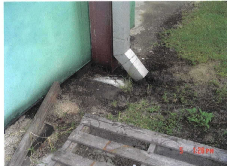
28. Outside of used oil storage area located in household hazardous waste drop off area
