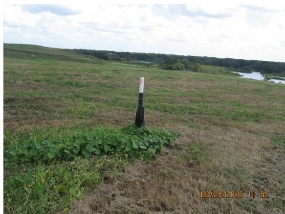
Phase II Piezometers
