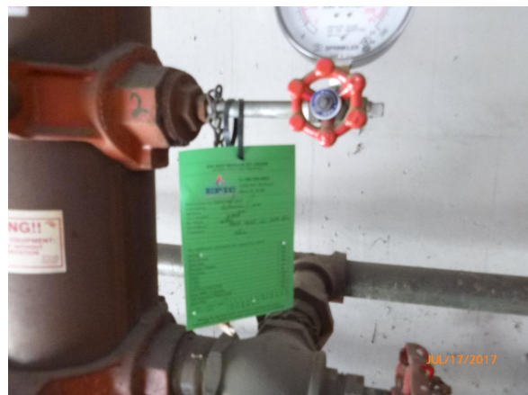
Fire equipment inspection tag.
