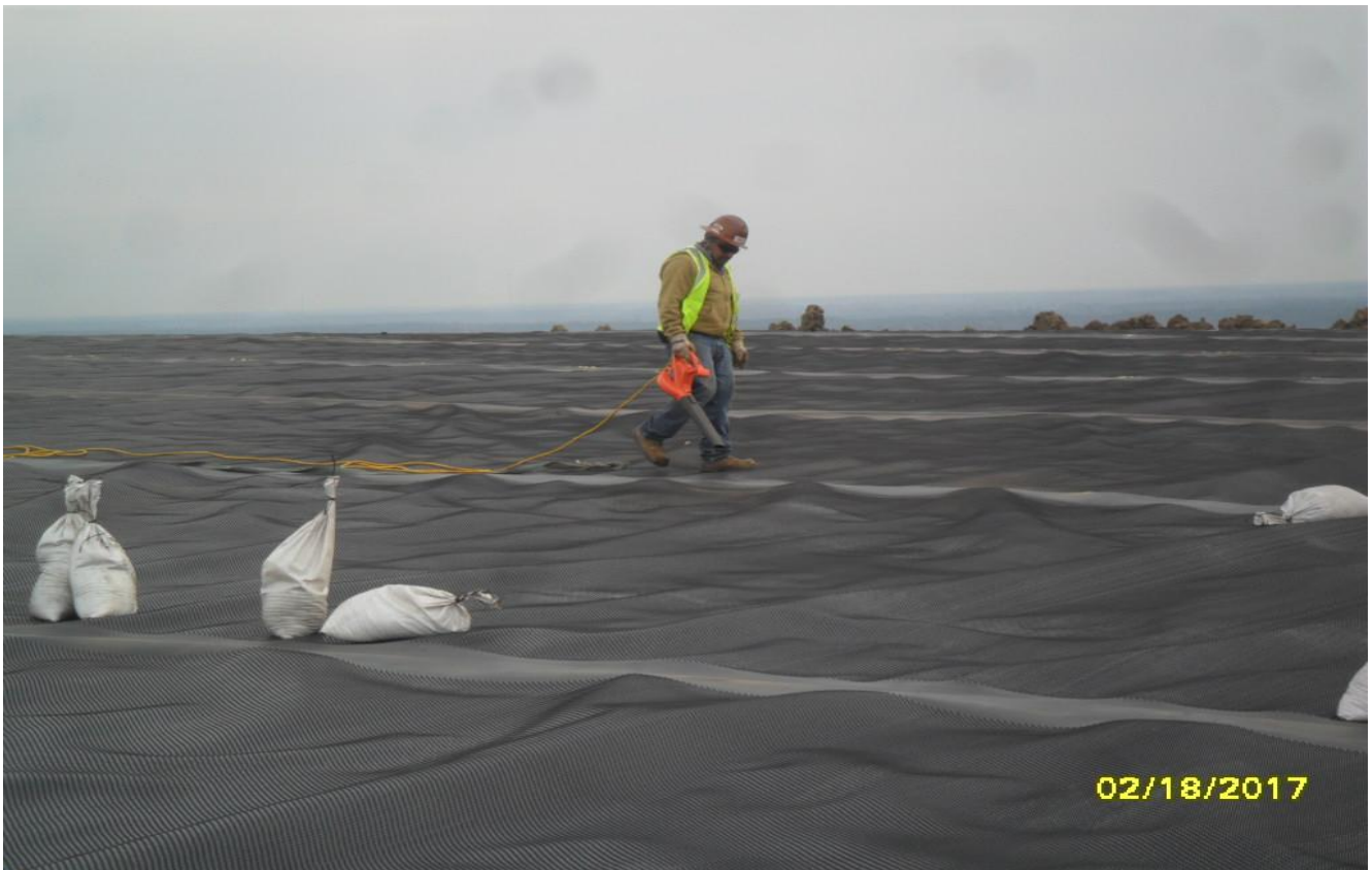
Cleaning geomembrane for geotextile placement at top of hill (facing Southeasterly) (February 2017)
