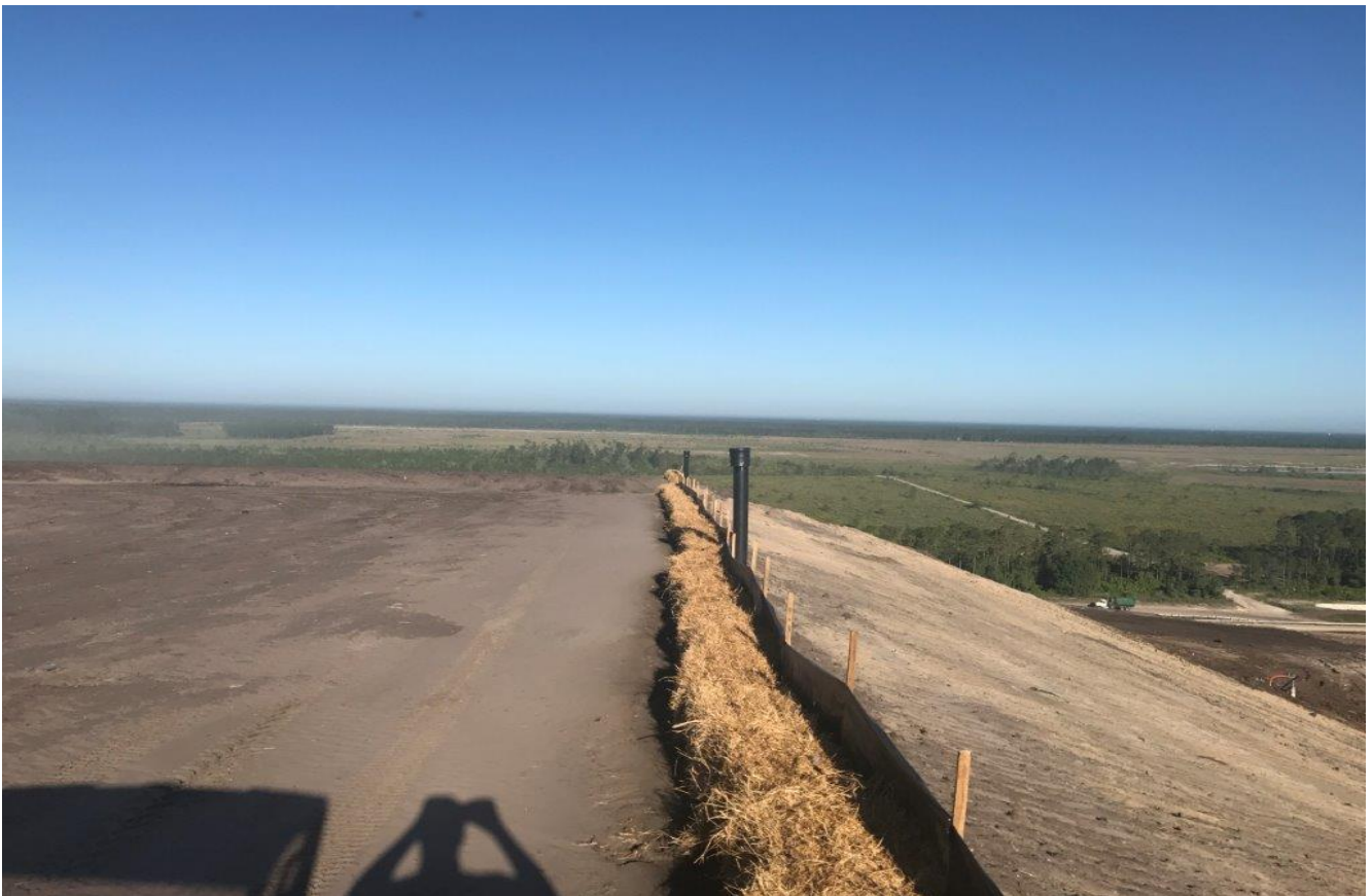
Edge of liner markers and haybales top of hill (facing Westerly) (May 2017)
