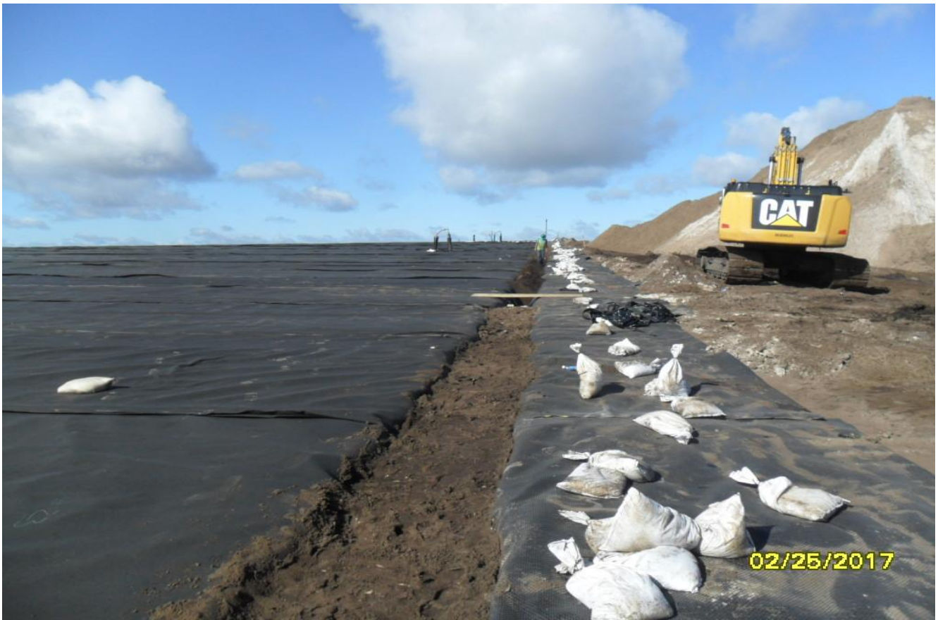
Filling temporary anchor trench at top of hill along Profile 3 (facing Westerly) (February 2017)
