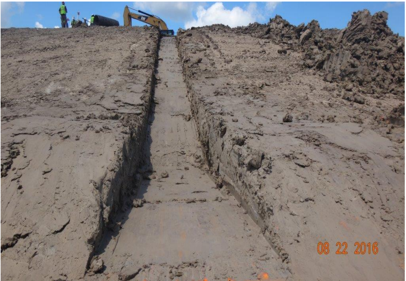
Compacting clay trench between Terraces 9 and 10 at downcomer D-27 (facing Westerly) (August 2016)
