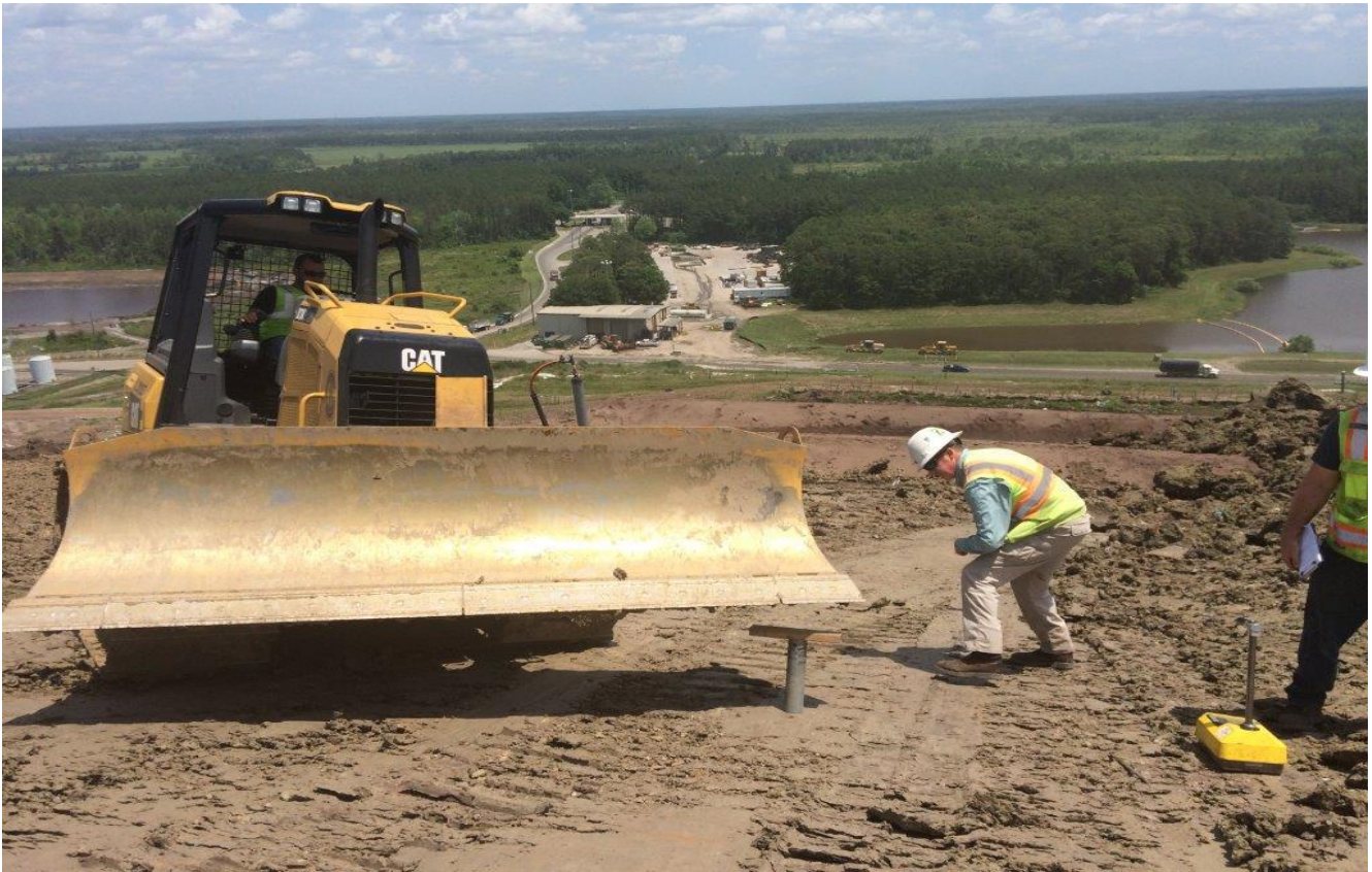
Pushing Shelby Tubes for the Permeability Testing – Clay Test Strip – Units 82-84 (Facing Easterly) (May 2016)
