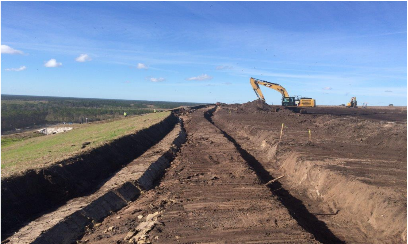
Exposing clay and constructing anchor trench at Terrace 10 Unit 87 (facing Southerly) (January 2017)
