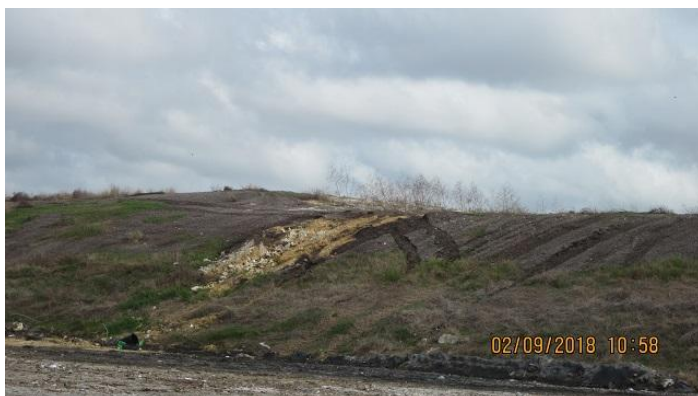
Erosion on Cell 5
