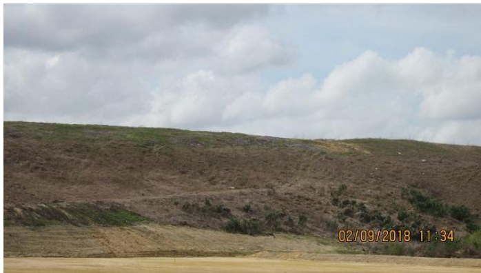
Damaged Cover on Cell 5
