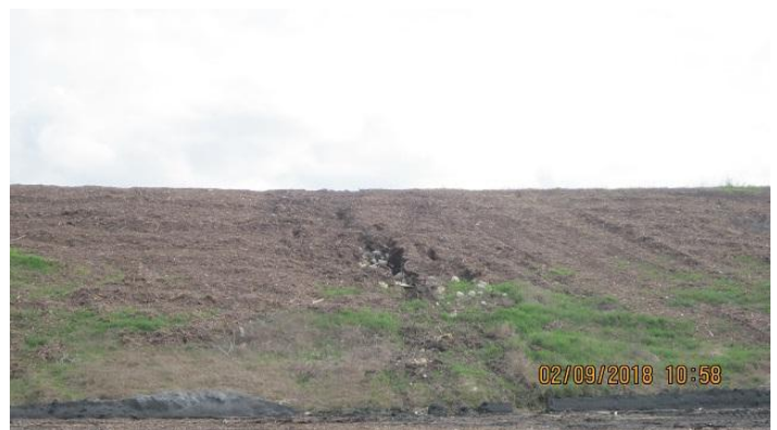
Erosion on Cell 4
