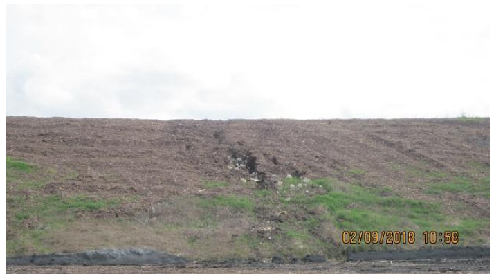
Erosion on Cell 4
