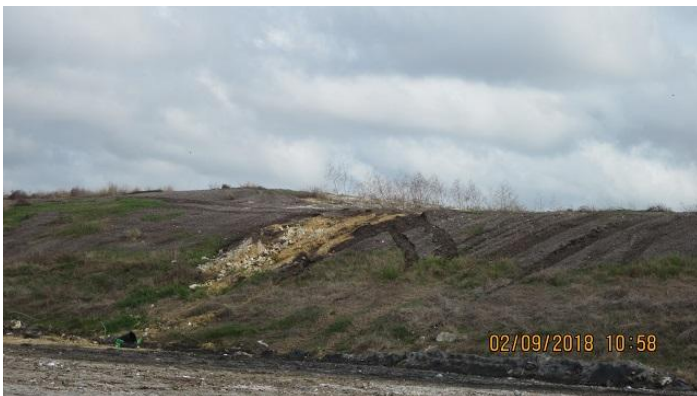
Erosion on Cell 5
