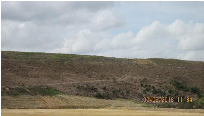
Damaged Cover on Cell 5
