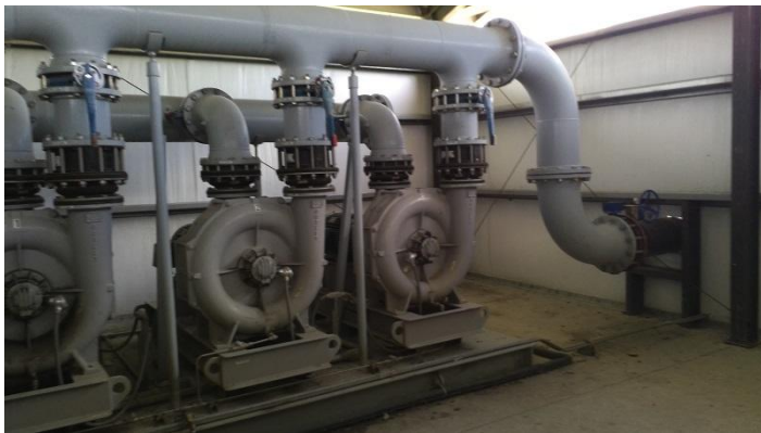
Gas Flare Blowers
