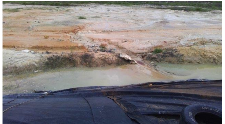
Runoff and Erosion
