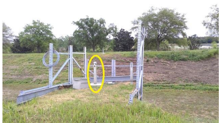
MW-6: Deficient Well Casing
