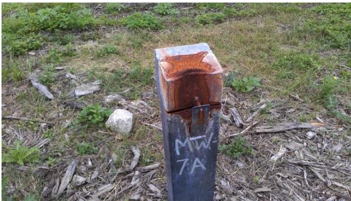
MW-7A: Missing Lock
