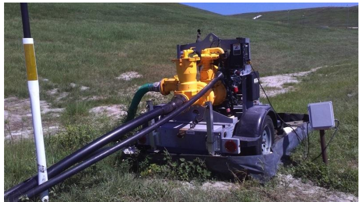
Temporary PS-2 In Use
