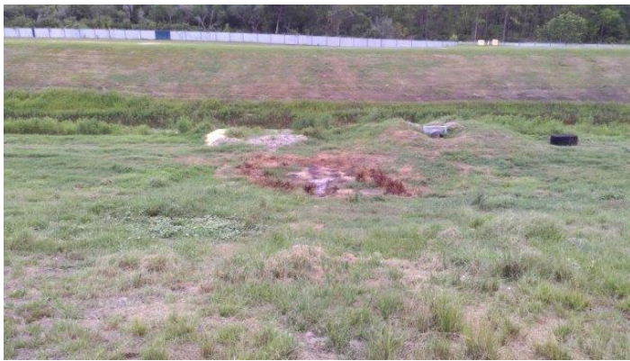
Seep on South-Facing Slope
