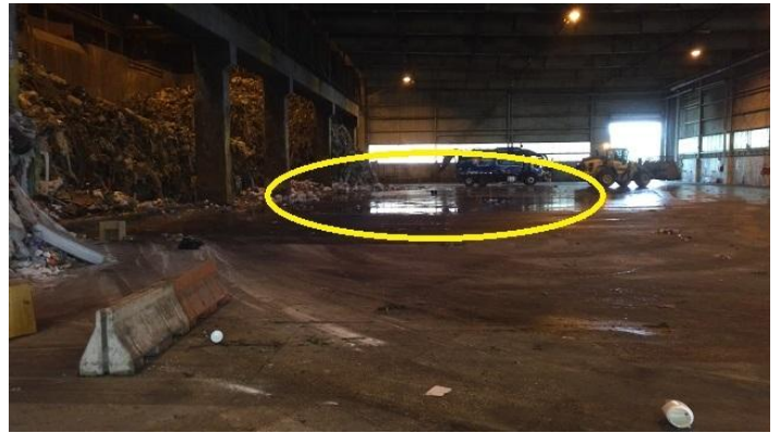
Minor Ponding - WTE Tipping Area
