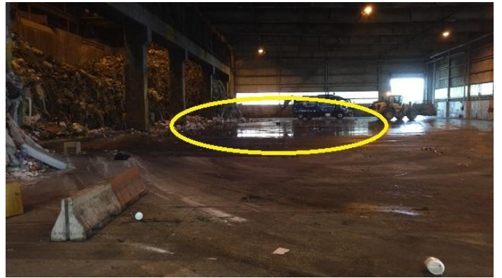
Minor Ponding - WTE Tipping Area
