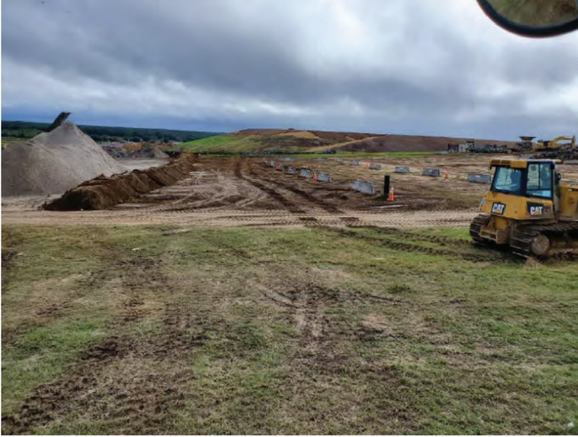
Tire Stockpile #3 with Fire Lane
