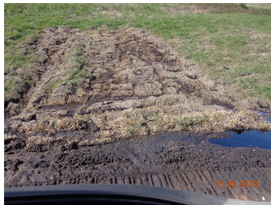
Leachate seep Cell 11
