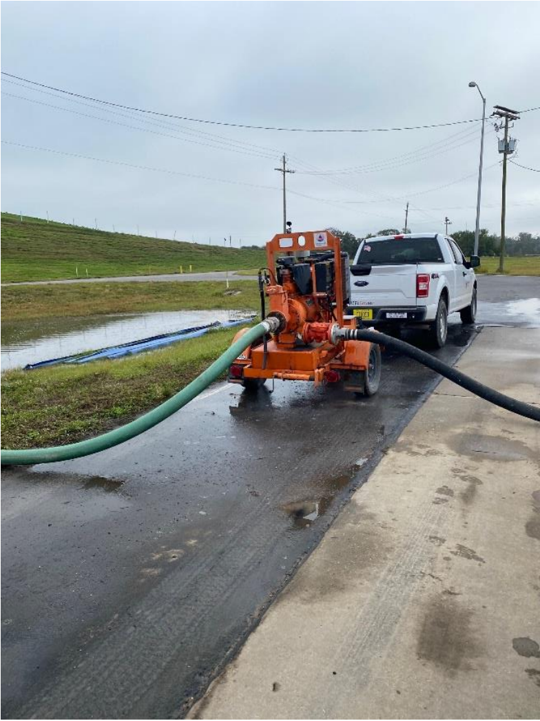
Photo 1. Affected area pre-cleanup (Looking NE)
