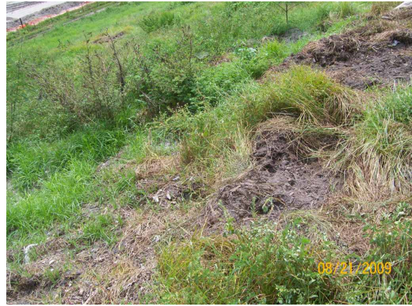
Excess veg and erosion on SSlope
