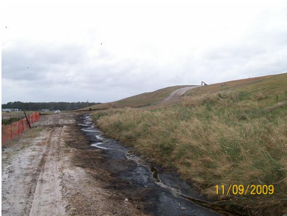
Leachate flowing on S side slope
