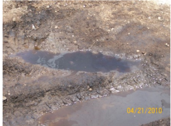
Leachate seep at toe of slope
