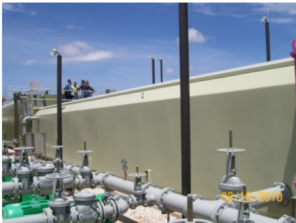
Chlorinated Effluent Tank
