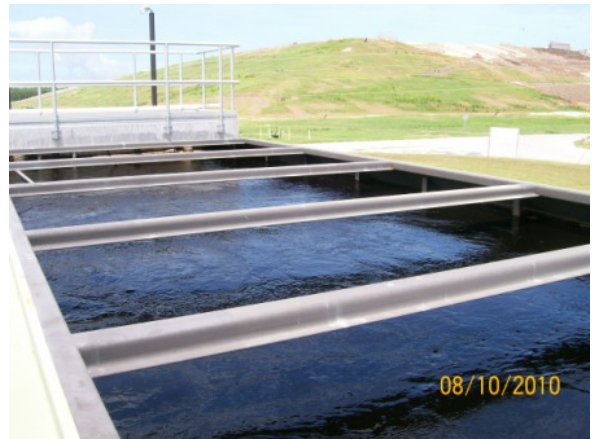
Leachate aeration tank
