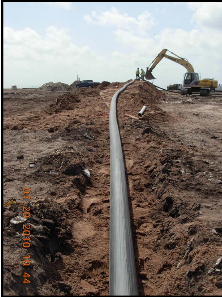
Photograph 54: Debris-free backfill soil used to maintain a minimum 5 percent slope for the temporarily above ground lateral to GW-15R.
