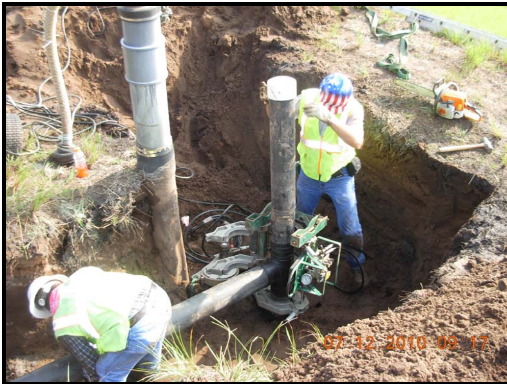
Photograph 32: Tie-in to GW-49 lateral riser for lateral to GW-50. Tie-in location above geomembrane skirt.
