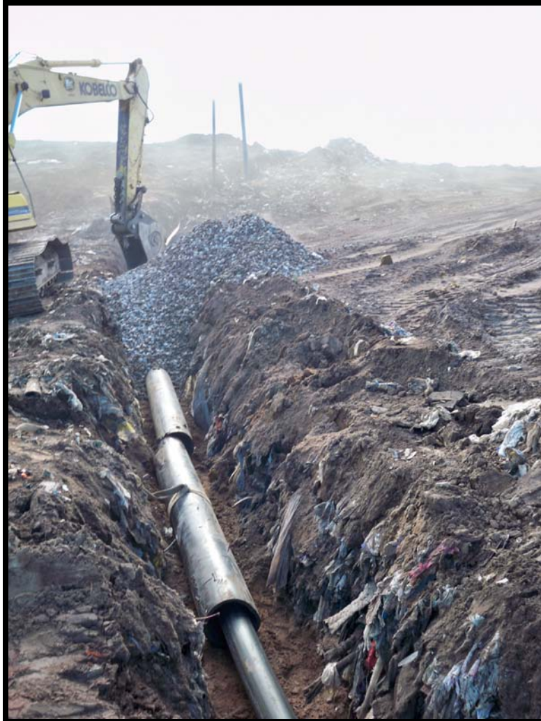
Photograph 68: Looking west, road crossing lateral trench going to GW-54. Backfilling road crossing with stone.
