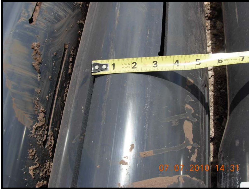
Photograph 5: 8" SCH 80 PVC 45° apart, staggered rows.
