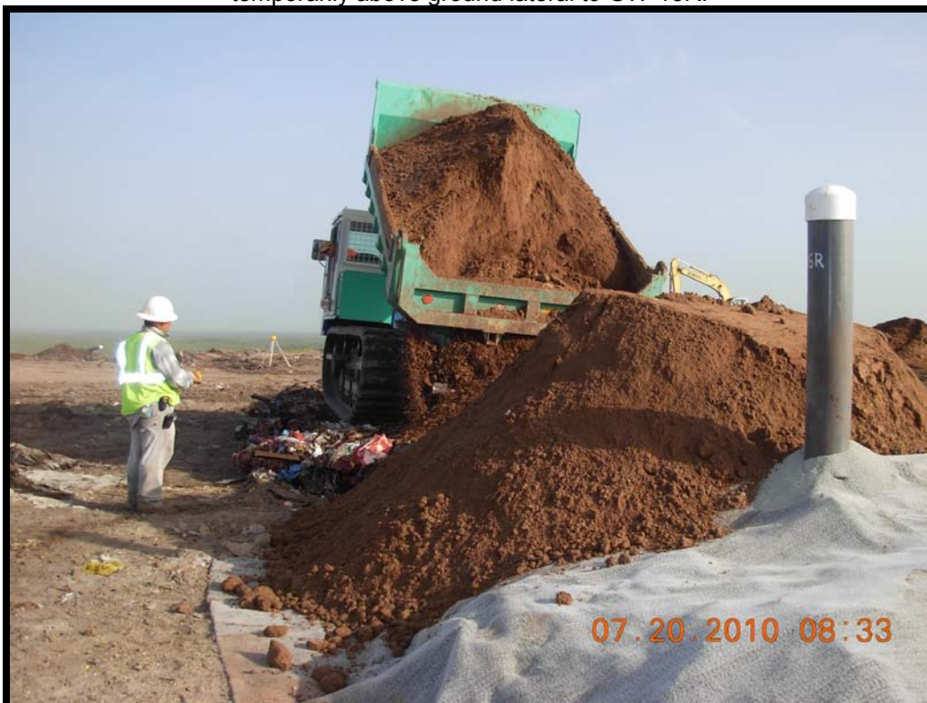
Photograph 52: Debris-free backfill soil placed over GCL sheet and trash used to maintain a minimum 5 percent slope for the temporarily above ground lateral to GW-15R.
