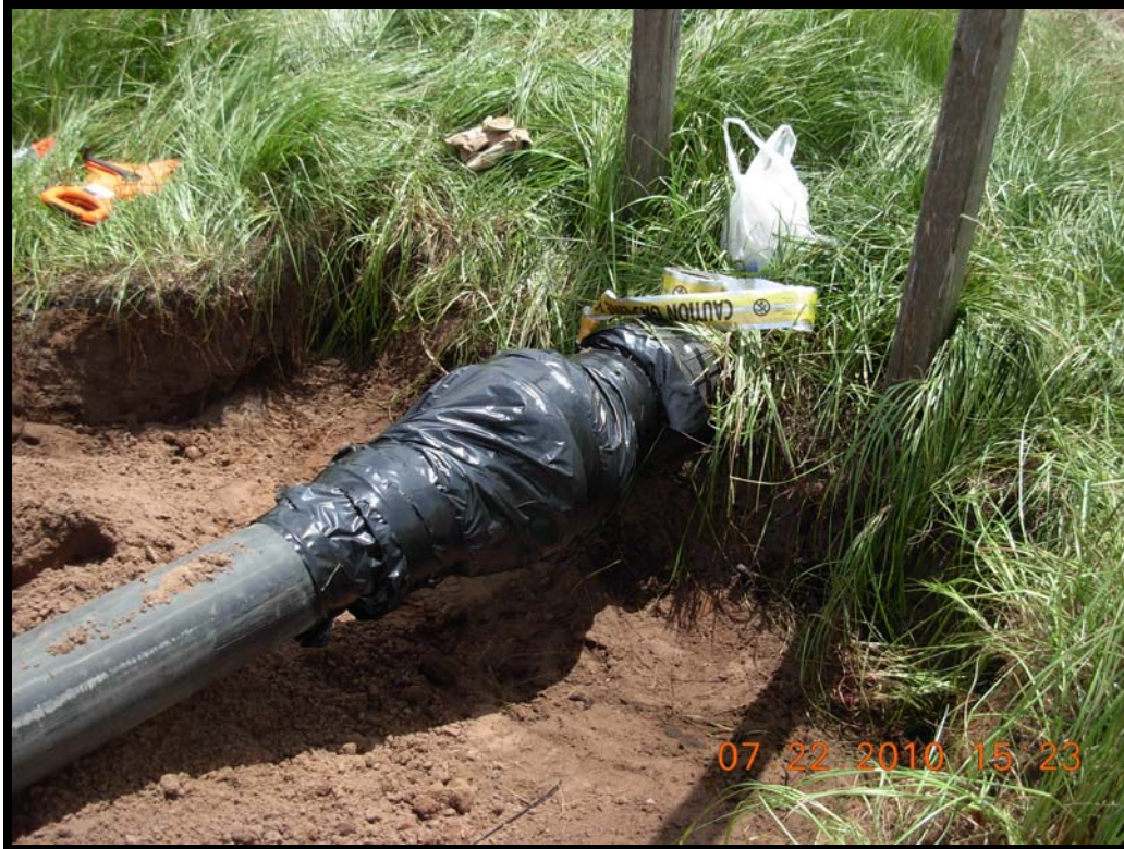
Photograph 58: Extraction well GW-35 lateral tie-in with 8" flange that reduces to 6" wrapped in plastic and duct-taped.
