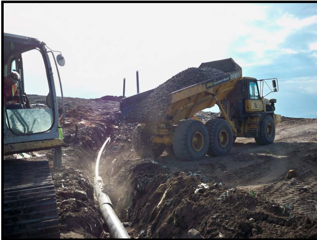
Photograph 67: Looking west, road crossing lateral trench going to GW-54. Backfilling road crossing with stone.
