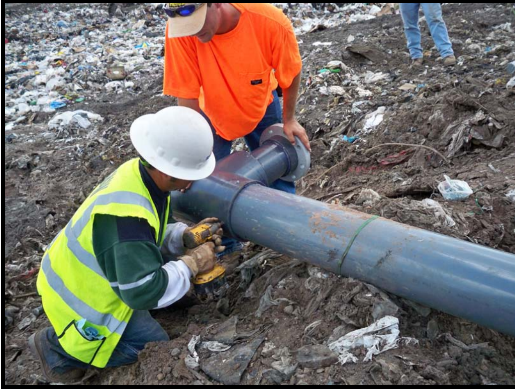
Photograph 63: Lag bolting 8" PVC tee at remote well GW-36 to provide additional support at joints.
