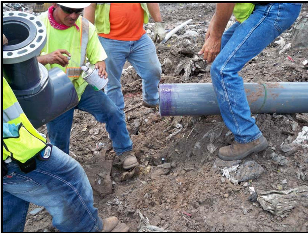
Photograph 62: Applying PVC primer and cement to 8" PVC tee at remote well GW-36.
