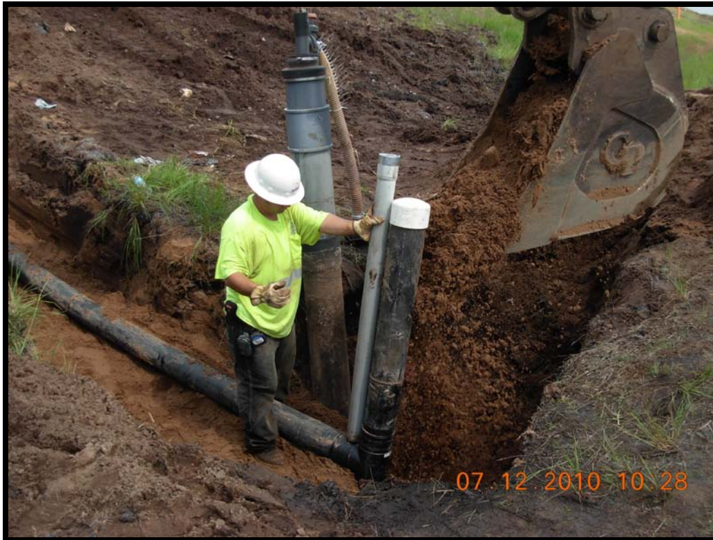
Photograph 34: Tie-in to GW-49 lateral riser for lateral to GW-50. Survey riser placed on top of top.
