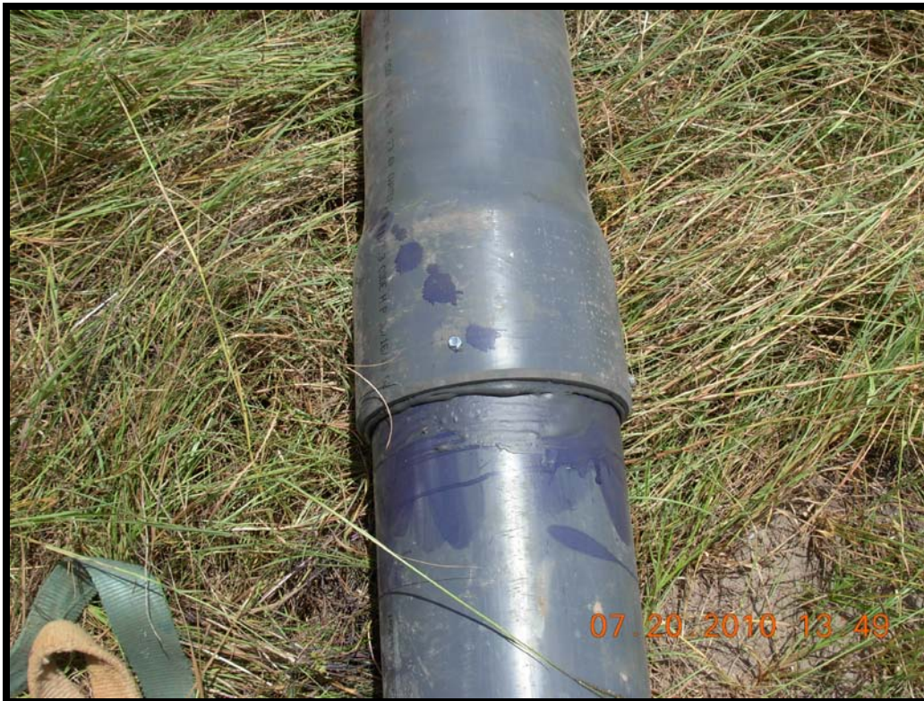
Photograph 48: PVC primer used prior to PVC cement when joining well casing joints. Self tapping screws used to supply additional support at each well casing joint.
