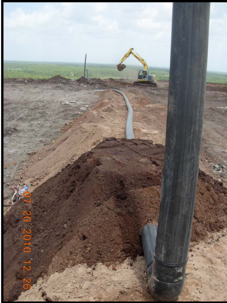
Photograph 55: Debris-free backfill soil used to maintain a minimum 5 percent slope for the temporarily above ground lateral to GW-15R.
