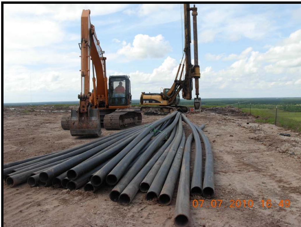
Photograph 2: 6" SDR 17 HDPE pipe inventory.
