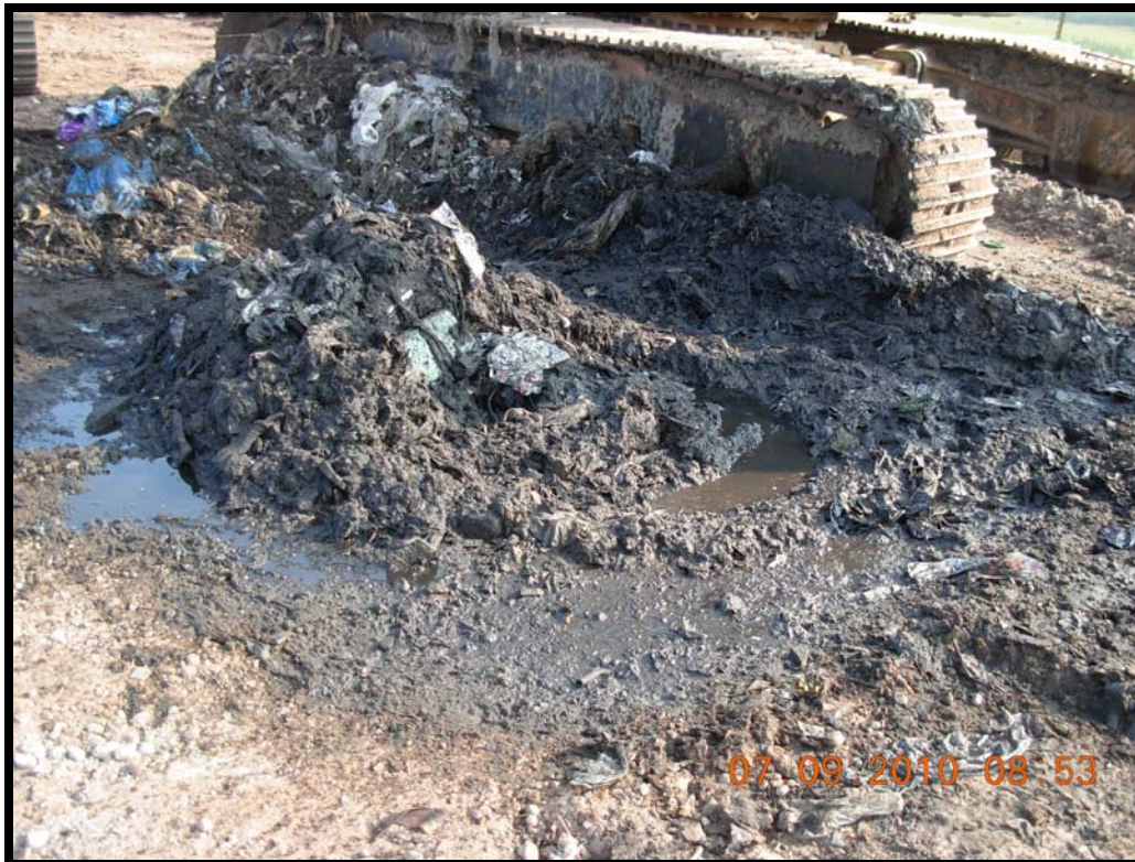
Photograph 24: Encountered saturated materials that could not be excavated using a bucket auger at GW-50.
