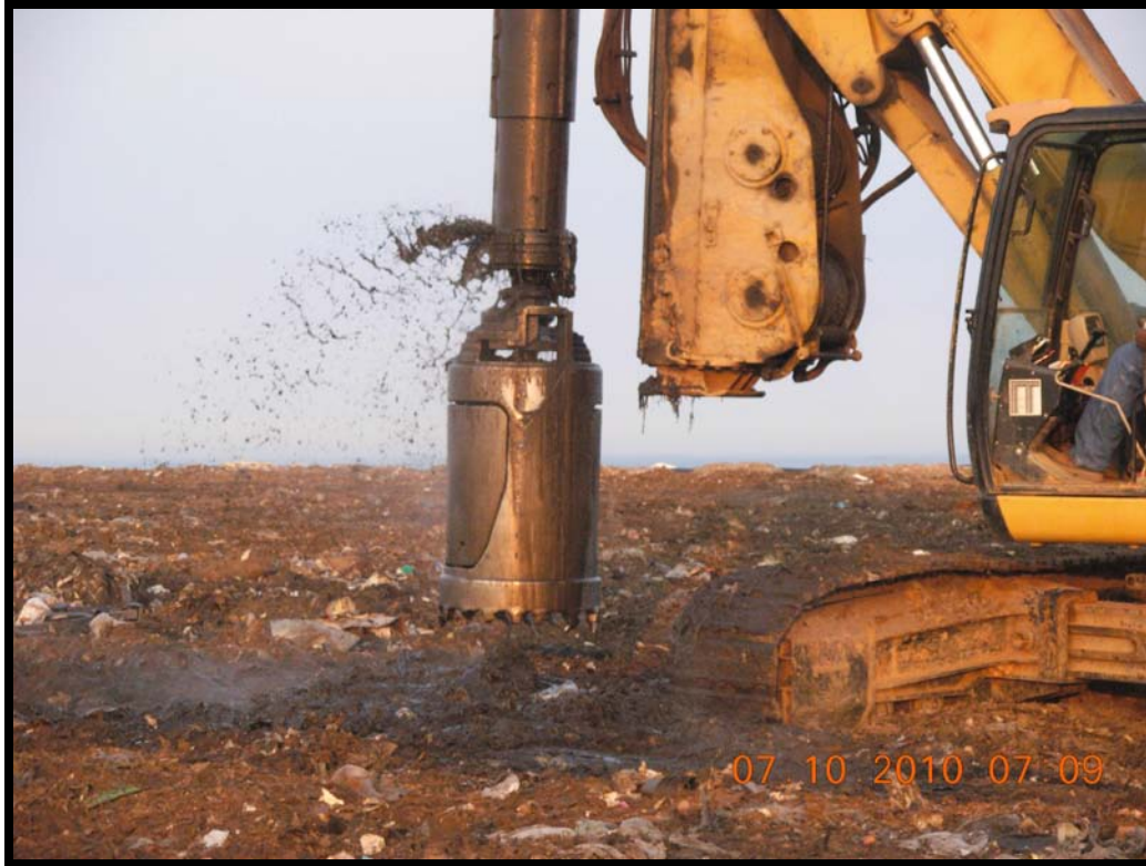
Photograph 31: Encountered saturated materials that could not be excavated using a bucket auger at GW-50.
