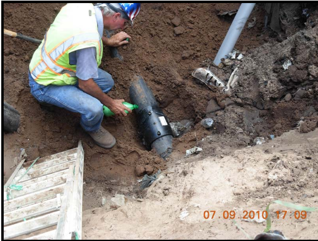
Photograph 29: Extraction well GW-45 lateral tie-in with 6" HDPE electrofusion coupling. Soap testing coupling – PASSED.
