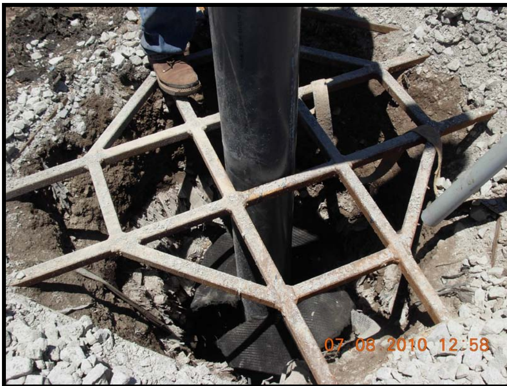
Photograph 18: Geotextile donut at extraction well GW-45.
