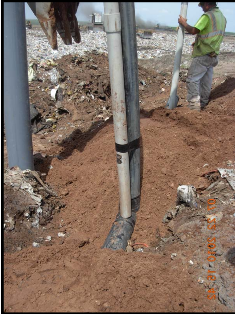
Photograph 60: Lateral riser to GW-35 with tee and 10 foot lateral stub-out for future tie-in with survey risers placed on top of pipe.
