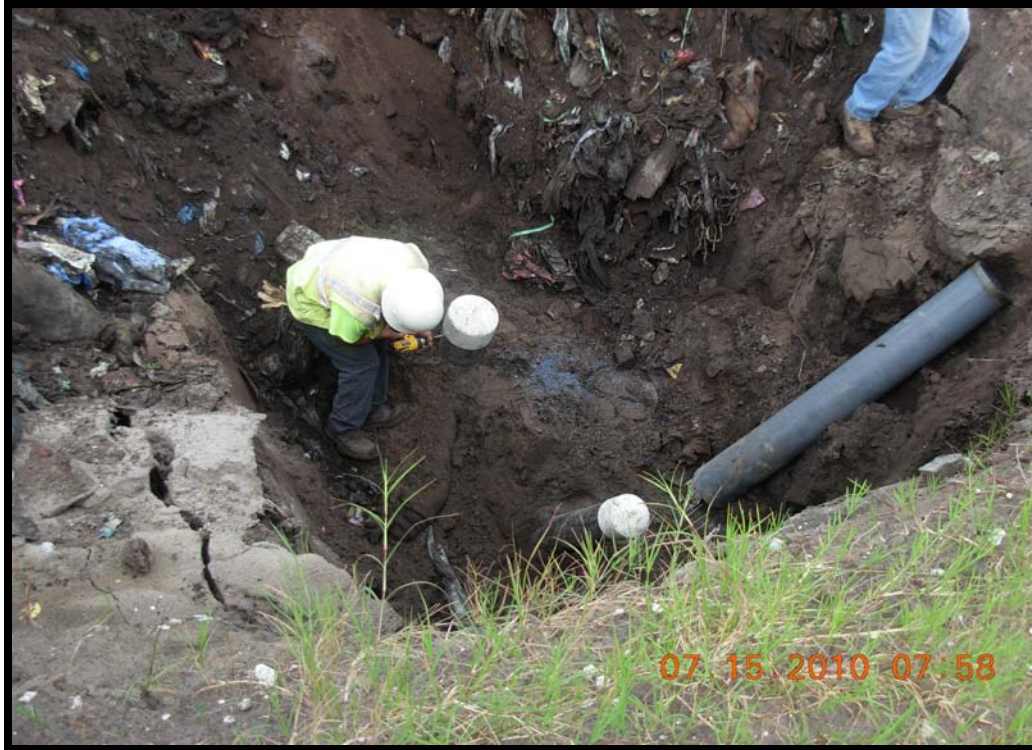
Photograph 42: Abandoned extraction well GW-4 and lateral riser.
