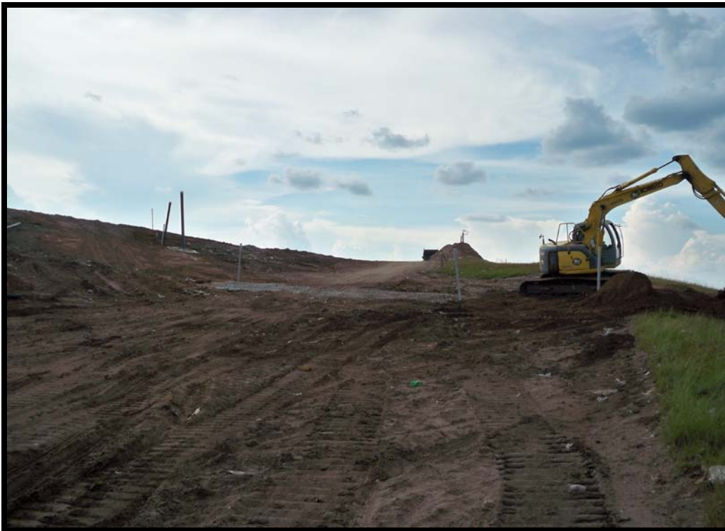
Photograph 70: Looking west, lateral road crossing going to GW-54. Backfilled road crossing with stone.
