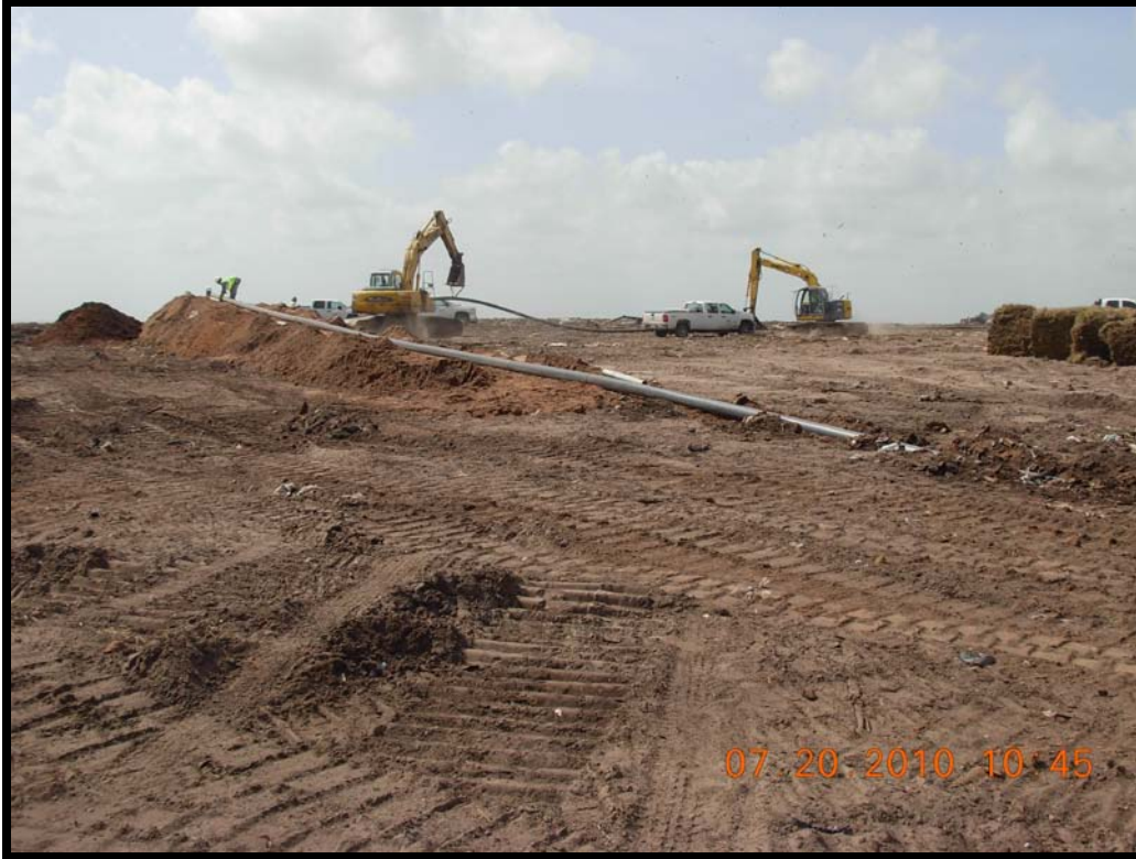
Photograph 53: Debris-free backfill soil used to maintain a minimum 5 percent slope for the temporarily above ground lateral to GW-15R.
