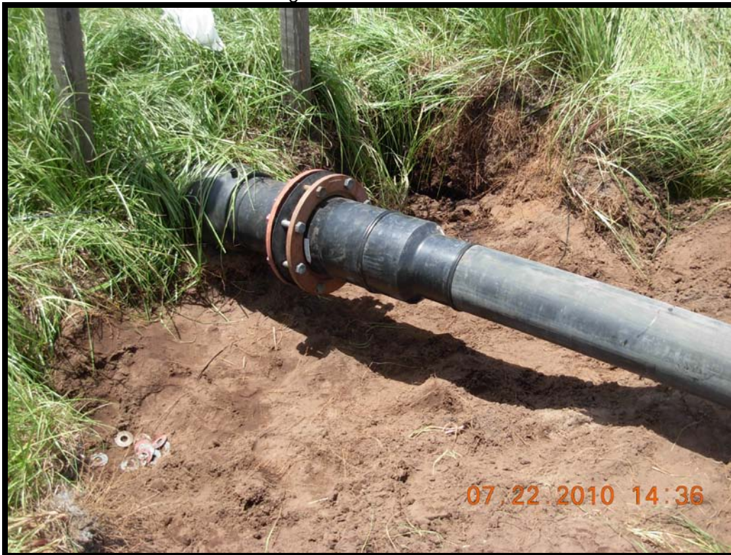
Photograph 57: Extraction well GW-35 lateral tie-in with 8" flange that reduces to 6".
