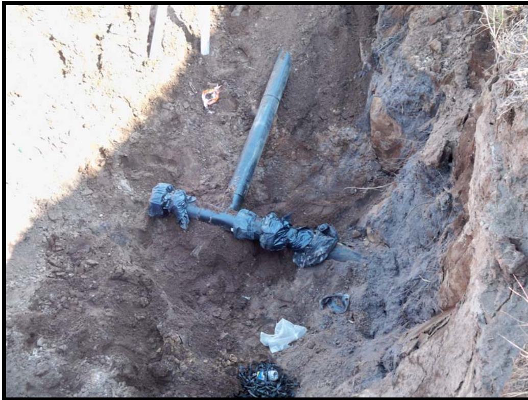
Photograph 71: Extraction well GW-60A lateral tie-in with 6" blind. 6" tee to 60R with 6" blind flange for future tie-in. Flanges wrapped in plastic and duct tapped.
