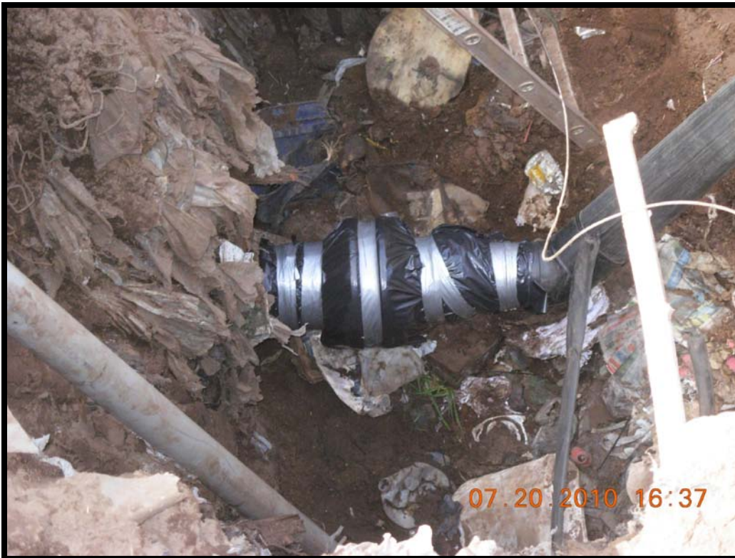
Photograph 50: Extraction well GW-27 lateral tie-in to existing 8" HDPE flange wrapped in plastic and duct-taped. 8" reduces to 6".
