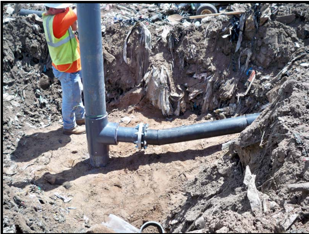
Photograph 64: 8" PVC tee at remote well GW-36. 6" PVC blind to 6" HDPE blind.
