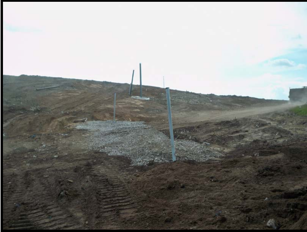
Photograph 69: Looking west, lateral road crossing going to GW-54. Backfilled road crossing with stone.
