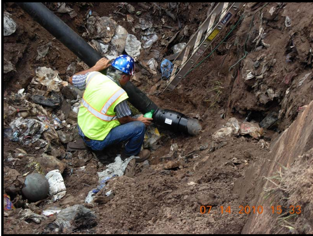
Photograph 40: Extraction well GW-4R lateral tie-in with 6" HDPE electrofusion coupling. Soap testing coupling – PASSED.
