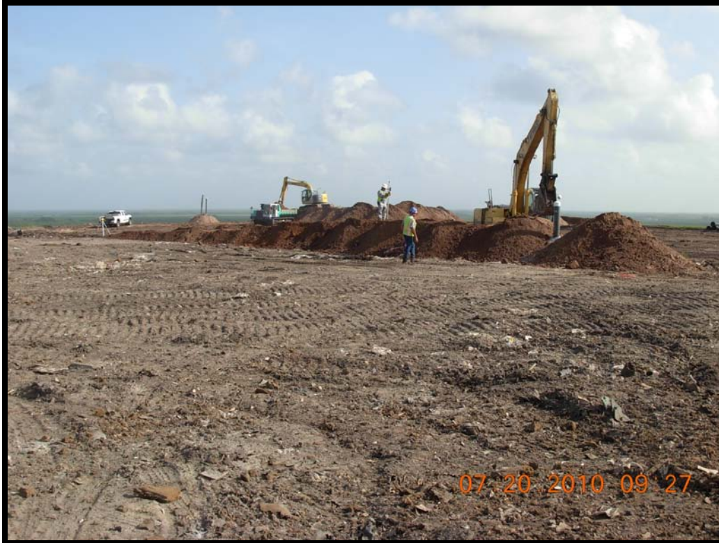
Photograph 56: Debris-free backfill soil used to maintain a minimum 5 percent slope for the temporarily above ground lateral to GW-15R.
