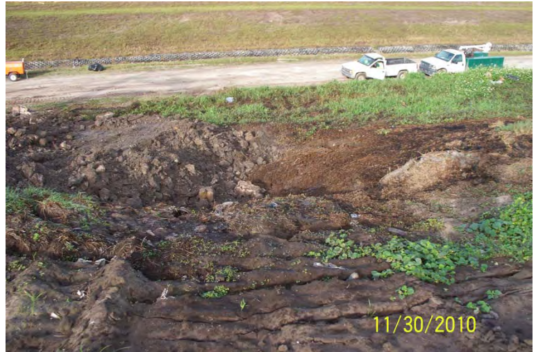
11/30/2010 Subsidence @ location of subsurface fire 100_0568.JPG
