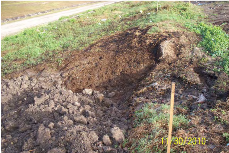
11/30/2010 Location of subsurface fire 100_0567.JPG
